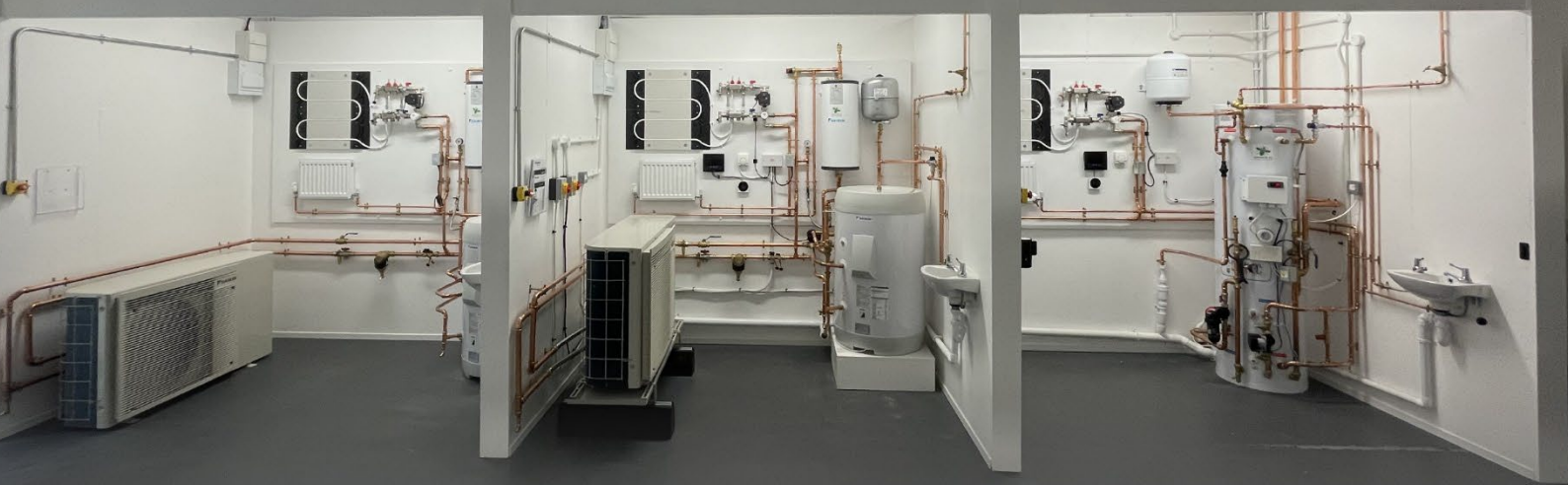
Quantum Renewable Training Facility Air Source Heat Pump Booth Set
